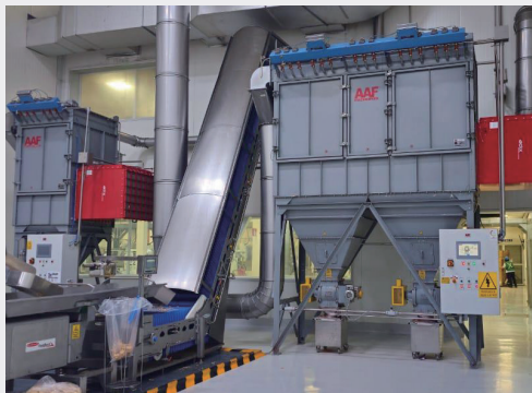
WONDAIR™ at Customer's Plant
